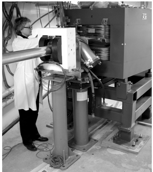
Fig. 185. The BL2A switching magnet in location.
