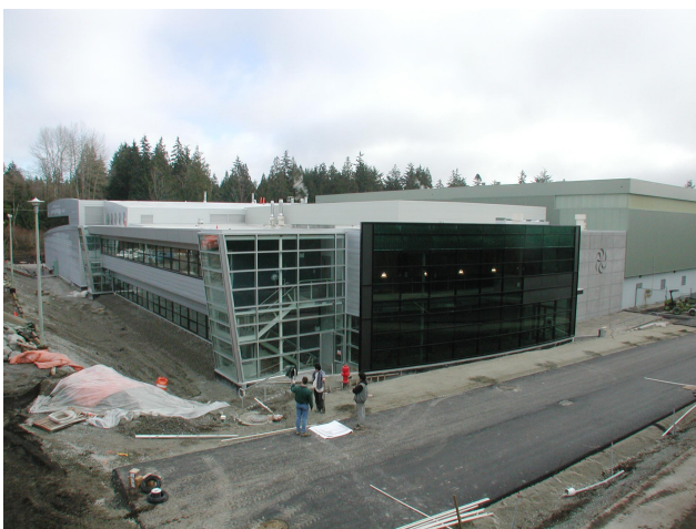
Fig. 217. A recent picture of the ISAC-II building. Landscaping is still in progress.
