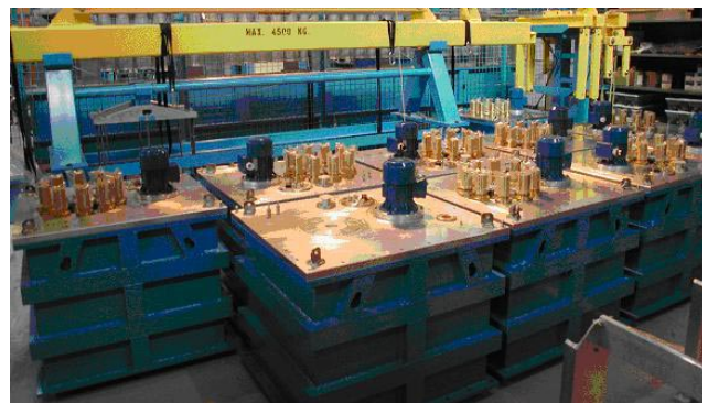
Fig. 251. View of some of the 20 assembled thyatron switch tanks at TRIUMF.
