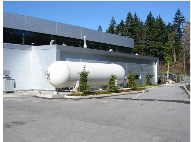
Fig. 245. He tank for the ISAC-II refrigeration system.
