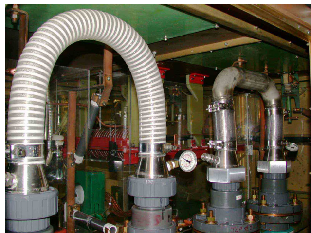
Fig. 188. Old and new (left to right) flexible couplings in the HVPS resistor cooling circuit.
