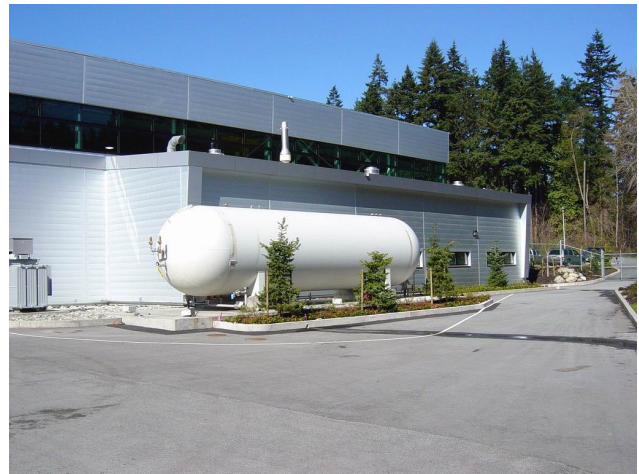
Fig. 245. He tank for the ISAC-II refrigeration system.
