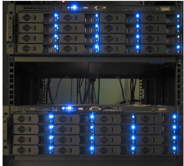
Fig. 145. Servers used for back-to-back and TRIUMF-CERN data transfers over a 10 GbE lightpath.
