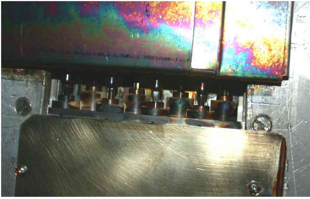
Fig. 257. Correction plate wire way insulators coated due to discharge.
