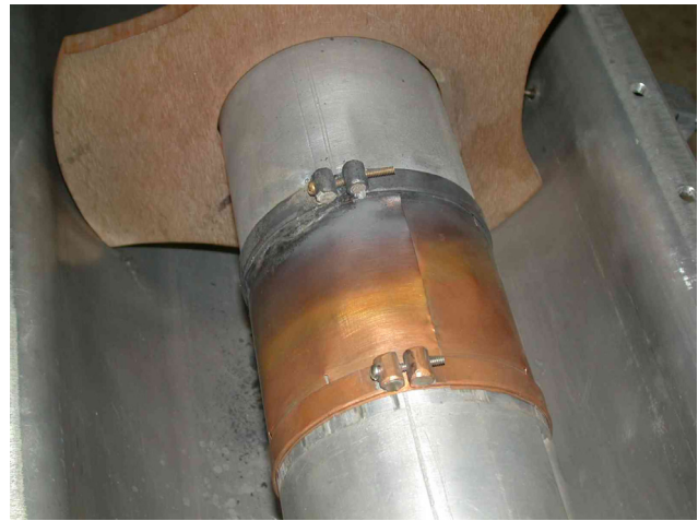
Fig. 256. Burnt spot at transmission line inner conductor joint.
