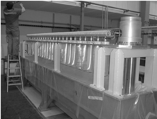
Fig. 162. Prototype PFN with capacitors and coil installed.
