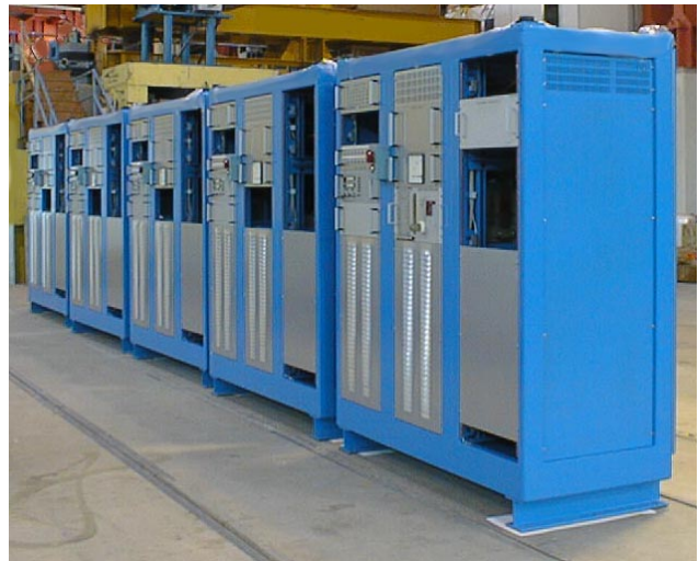
Fig. 173. Production series of 66 kV RCPSs near completion.
