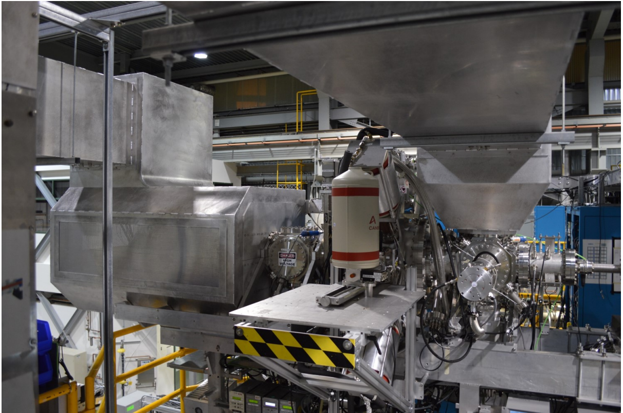
(a) Gun and collector ducts and gun enclosure.
