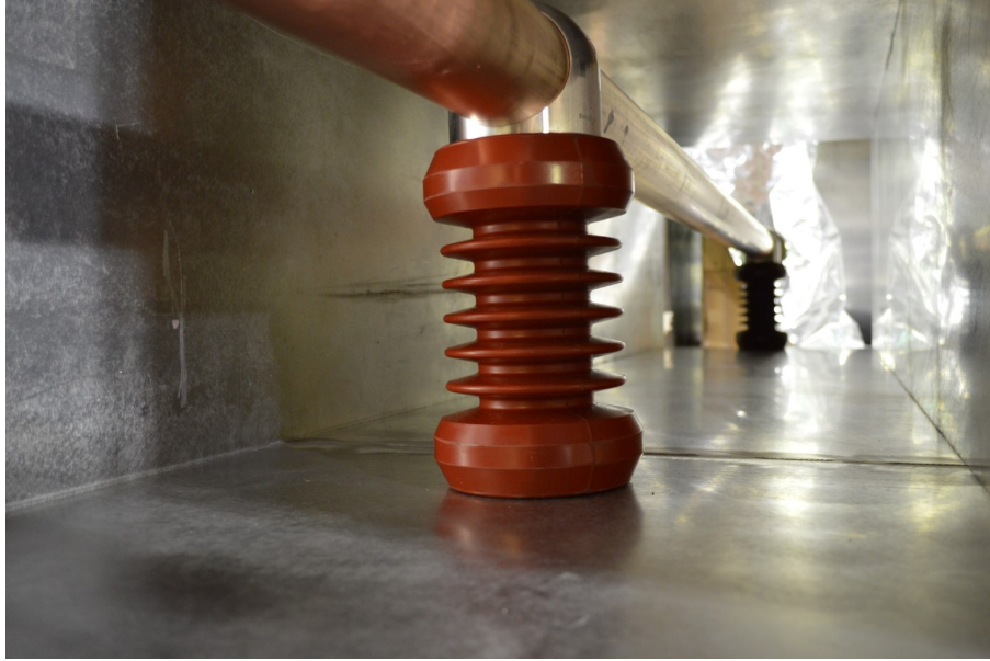
(a) Duct interior with pipe, insulators and endcaps.
