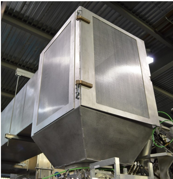
(b) Collector enclosure.
